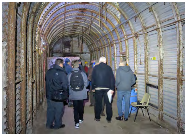
Exit passage from the Fort Southwick WWII tunnels, showing the steel reinforcement and corrugated iron lining – all in good original order.
